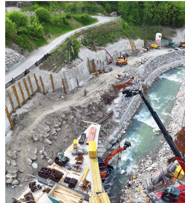
Hydroelectric Power Plant, Wagrain, Austria
