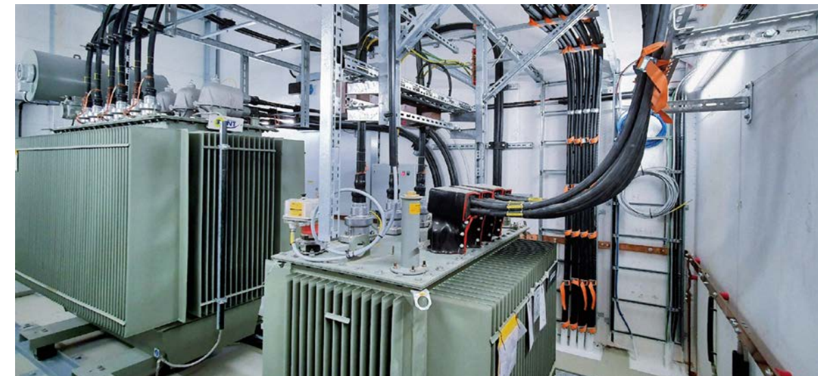
Electrical Installation, Töging Power Plant, Germany
